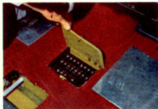
CIRCUIT BREAKERS are easily accessible through hatch in cabin floor, can be pulled to OFF position if desired.
